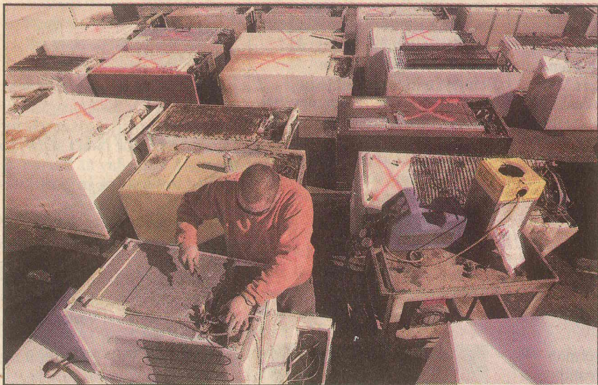
Robert Gallego empties freon from refrigerators that have been dropped off at the recycling yard. The orange 'X's' indicate units that have been processed.
